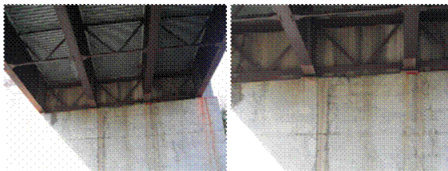
Potential Locations for AE Sensor Installation on the Bridge And the Back Wall.
